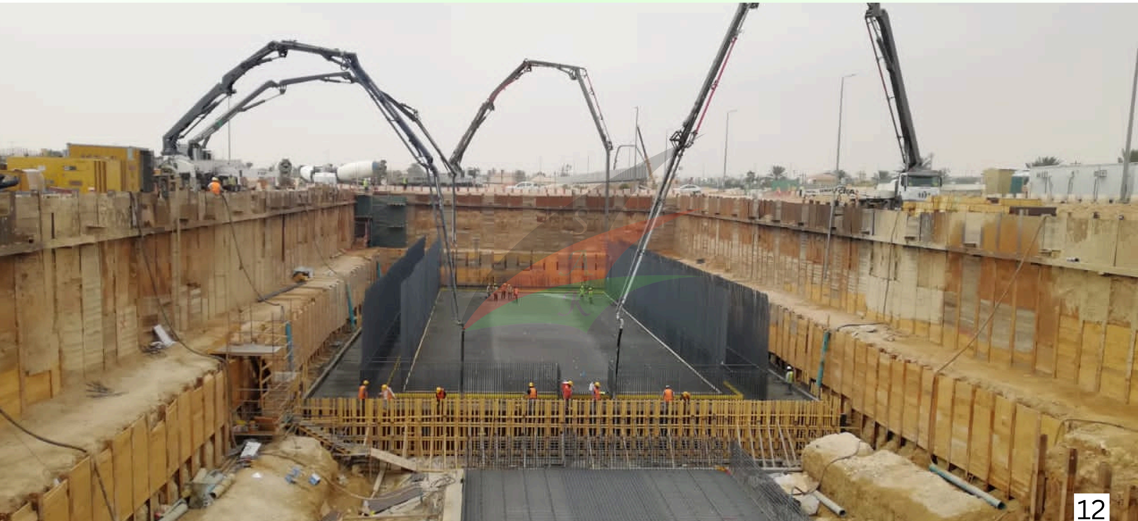
3700m 2 Stormwater tank in Buraydah project
