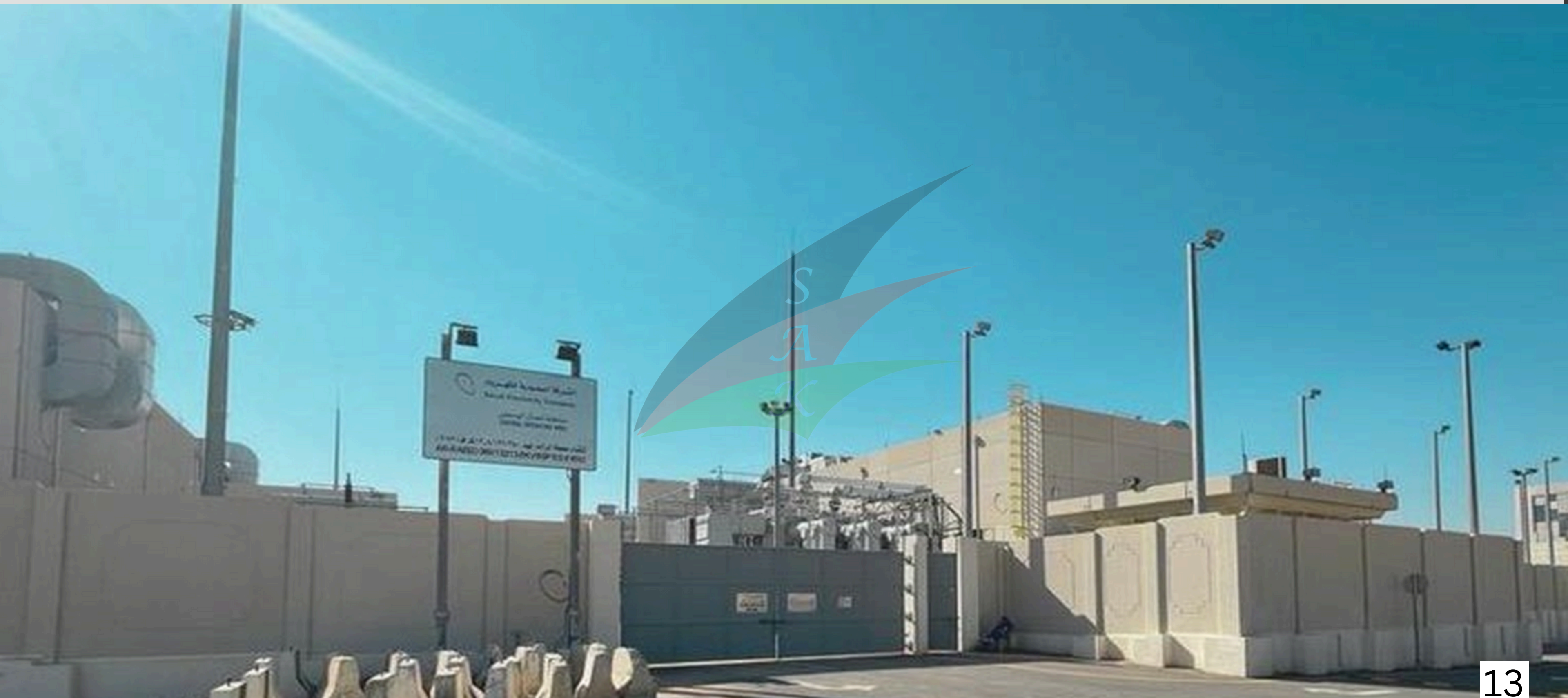
ArRaeed substation (380/132/13.8kV) SS#9042
